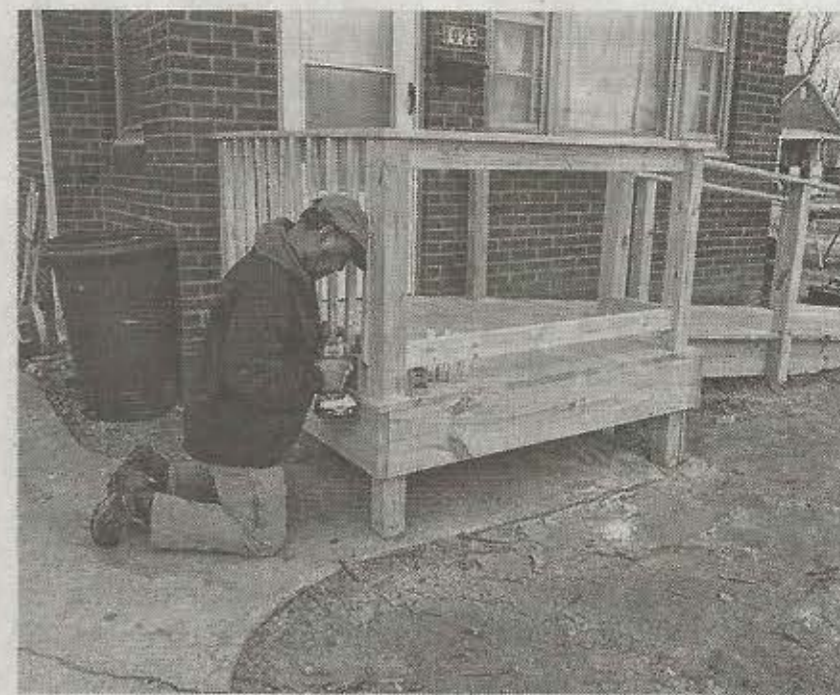
The homeowner at this location in Madison was able to get out of her house without assistance for the first time in about a year after Rebuilding Together Southwest Illinois finished this wheelchair ramp.
