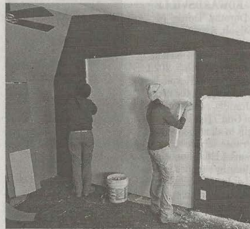
Volunteers from Rebuilding Together Southwest Illinois work on a project at a home in Granite City.
