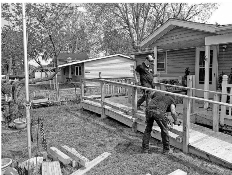
Volunteers from Phillips 66 finished a Rebuilding Together Southwest Illinois wheelchair ramp project April 18 in Madison.
